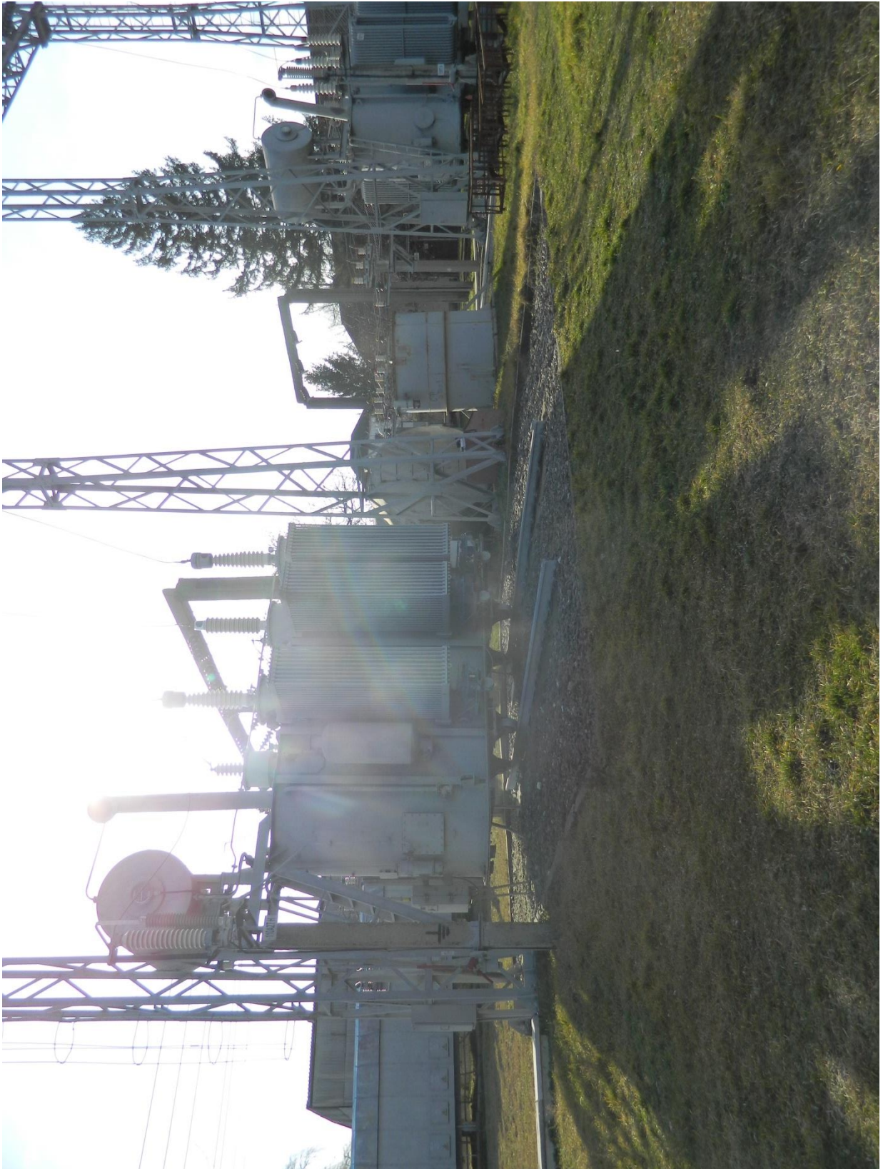
6. Existing transformer 110 kV side view.
