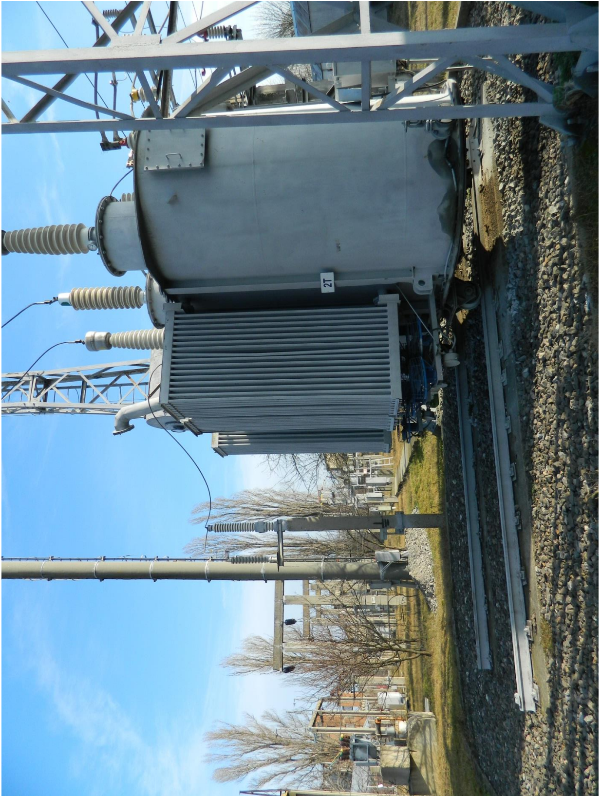
5. Existing transformer 110 kV side view.
