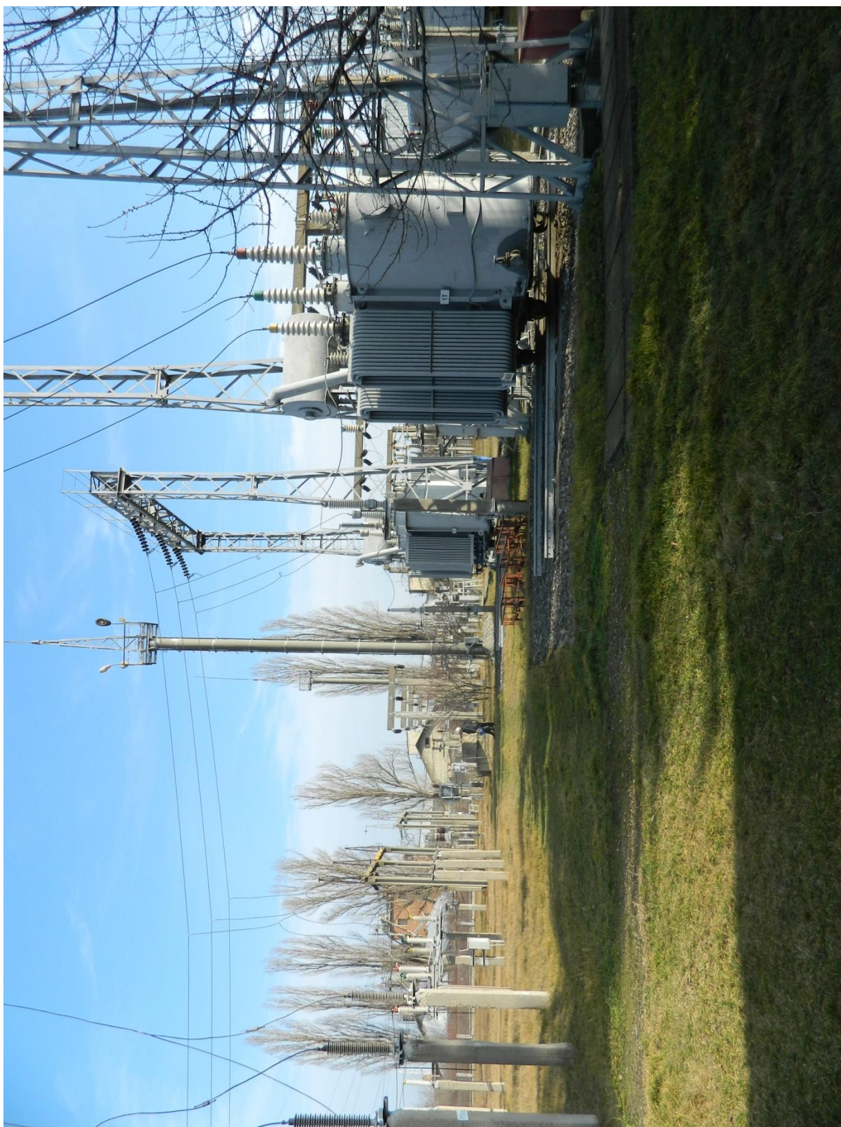
4. Power transformer area, view from the substation access gate
