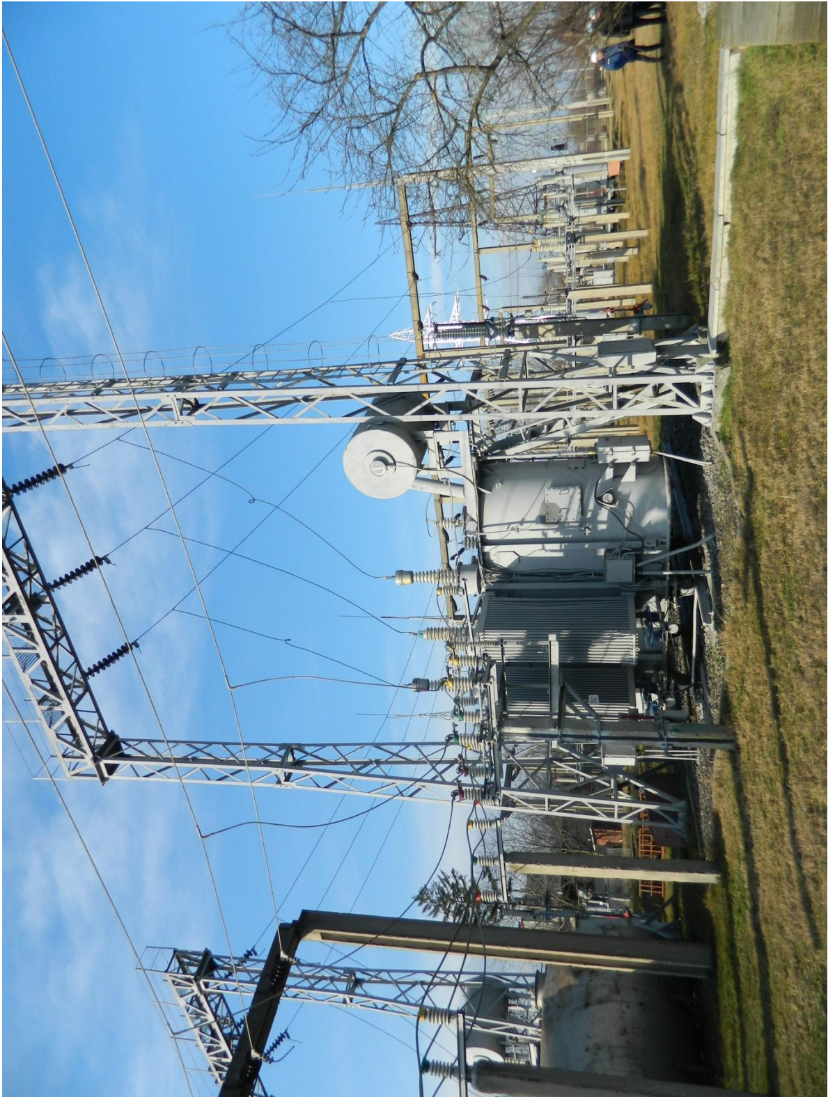
3. Existing transformer 35 kV and 10 kV external connections
