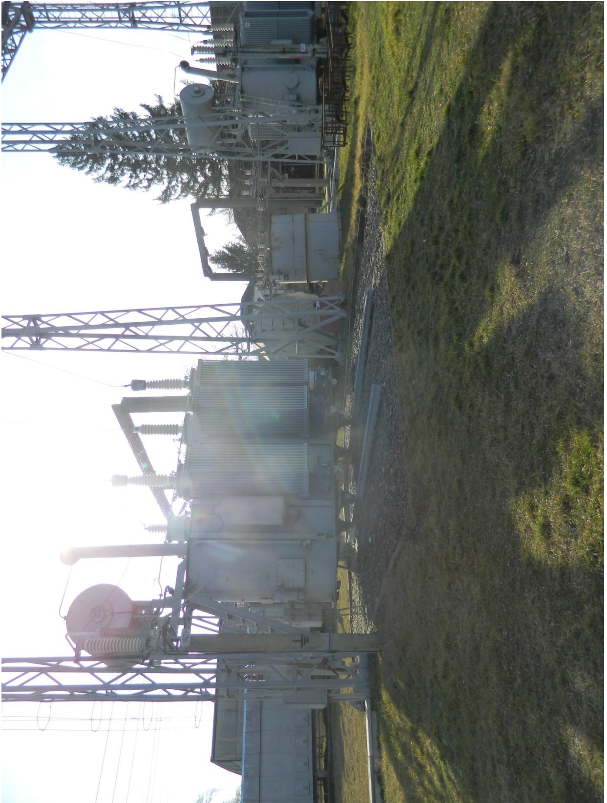
6. Existing transformer 110 kV side view.
