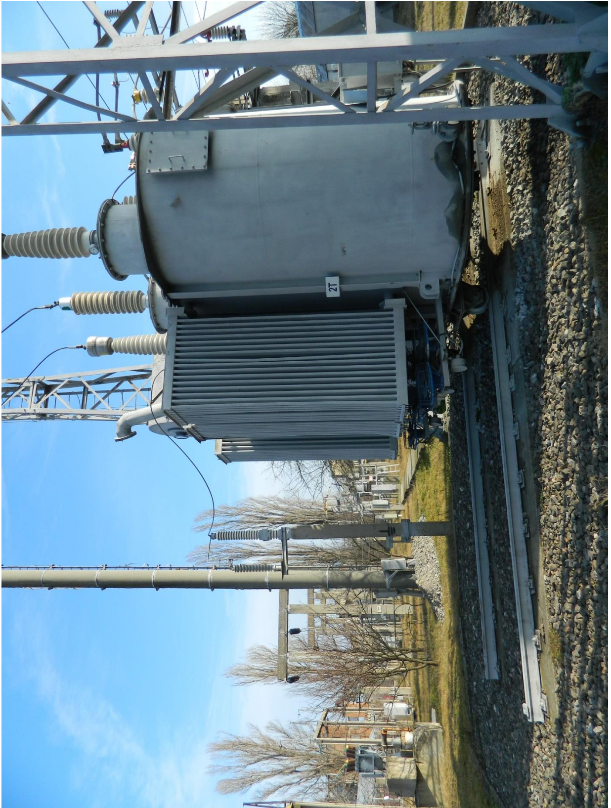
5. Existing transformer 110 kV side view.
