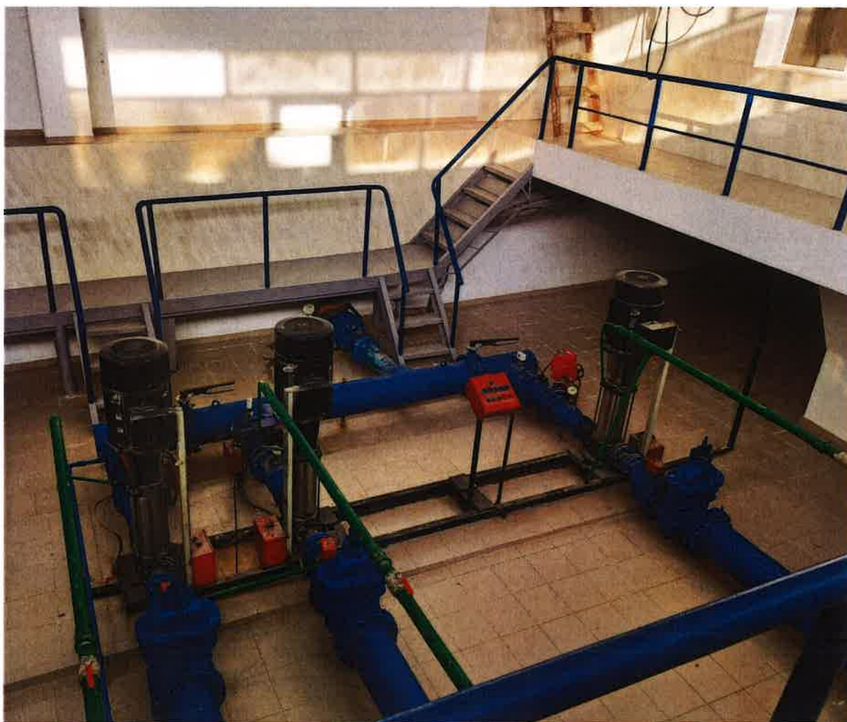
Figura 3.3. Nod hidraulic existent (SP-5)
