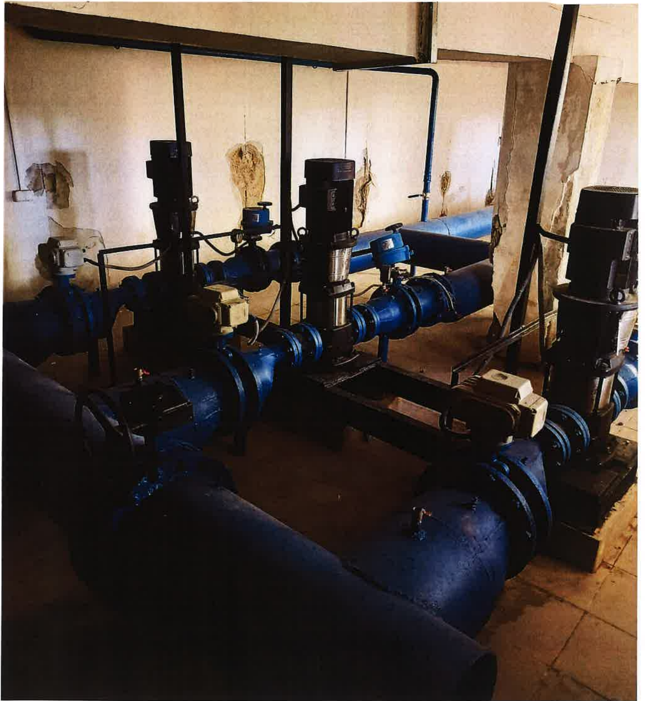
Figura 3.16. Nod hidraulic existent (SP-2)
