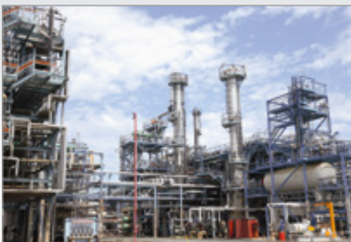
Refinery equipment (option)
