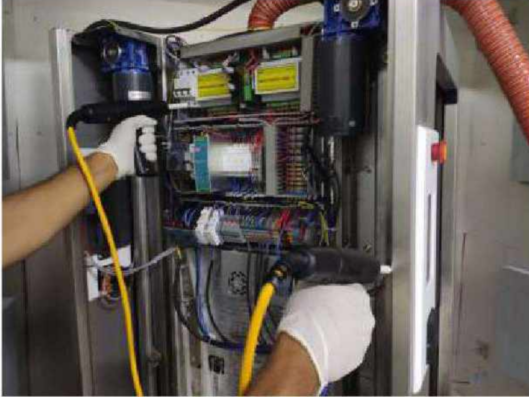
Photograph 13: Dielectric Strength Test
