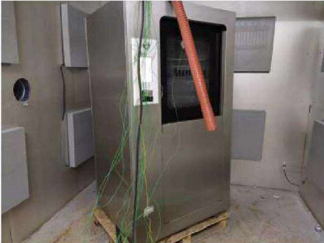
Photograph 15: Temperature Rise Test
