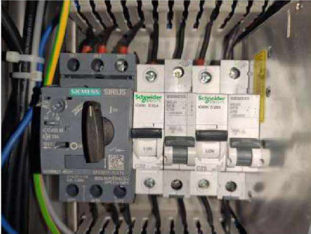
Photograph 3: Motor Switch and MCBs
