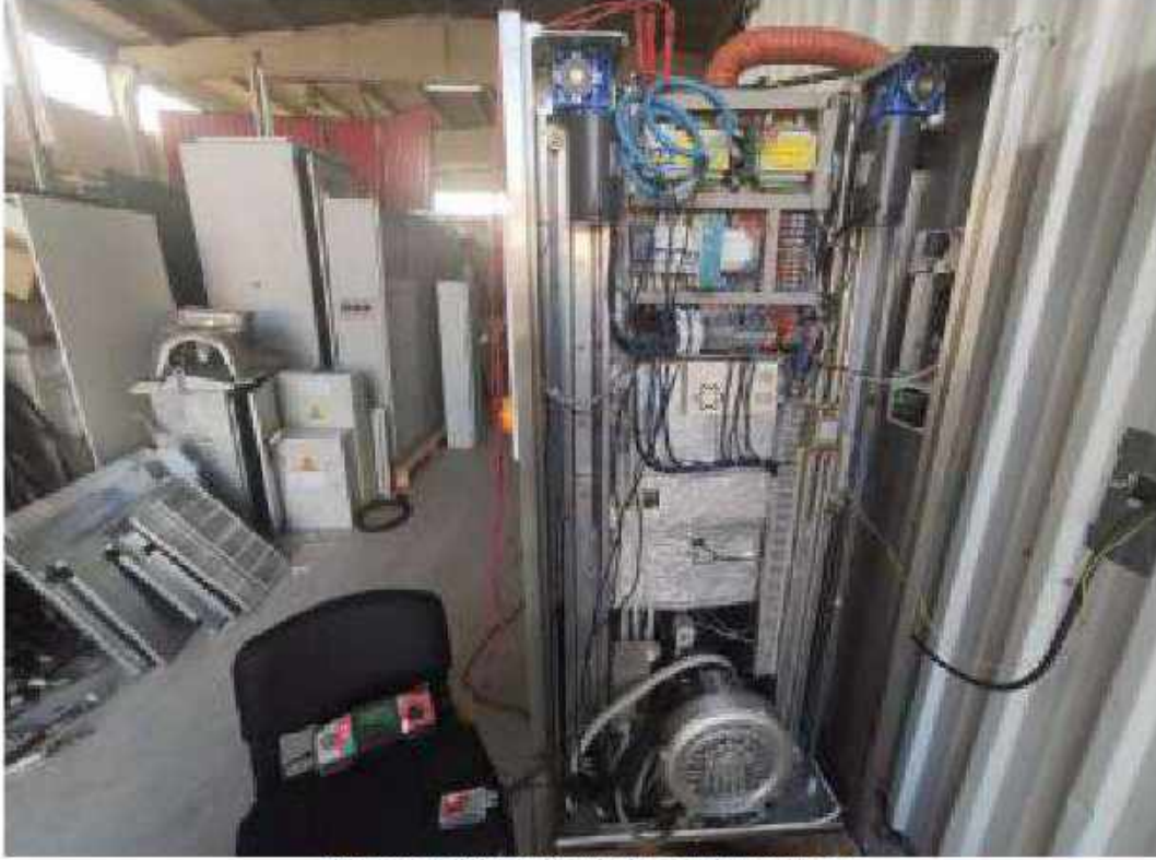
Photograph 15: Working Voltages Measurement
