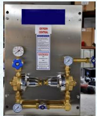
Manual Control Panel without Alarm
