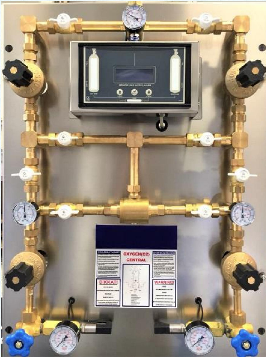
Automatic Control Panel of 30 m3/h Capacity
