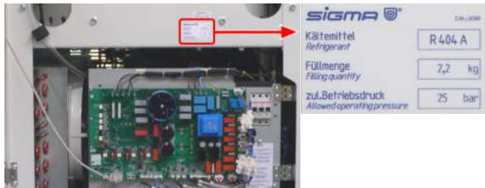
Fig. 29: Information concerning the filling quantity and type of refrigerant
