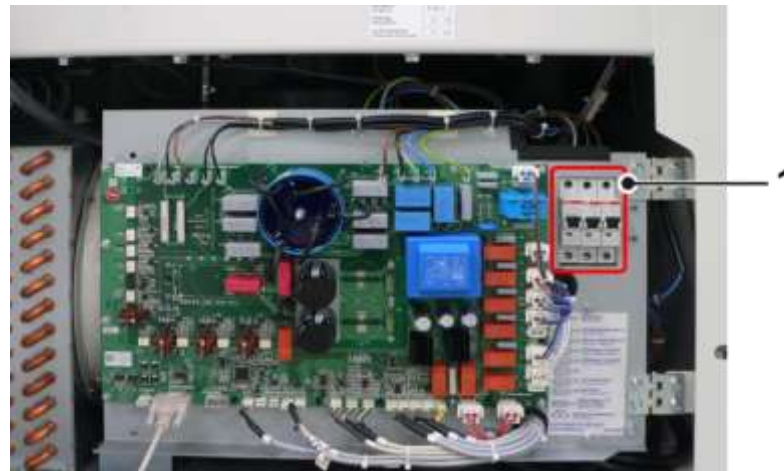
Fig. 24: Automatic circuit breakers
