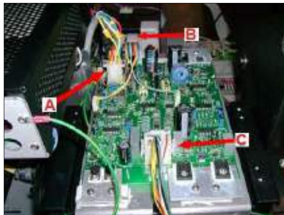
Figure 189: Generator Control Board
