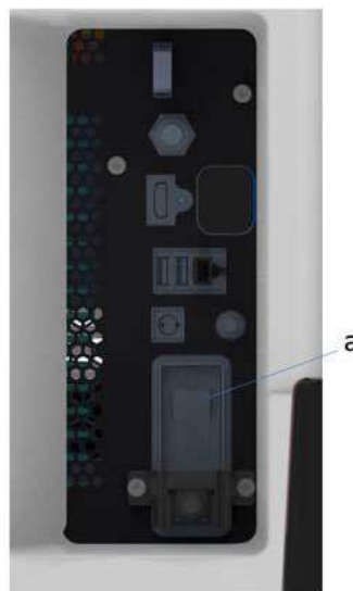
Figure 3-27. Circuit Breaker (located on the rear panel)
