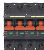
2 x 2 pole Breaker for each Battery string
