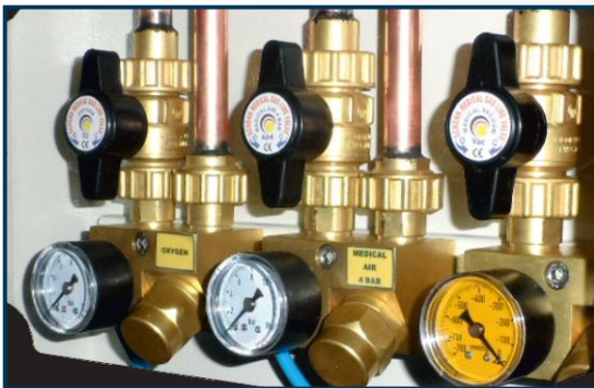
Zone Wall Unit Inside View
