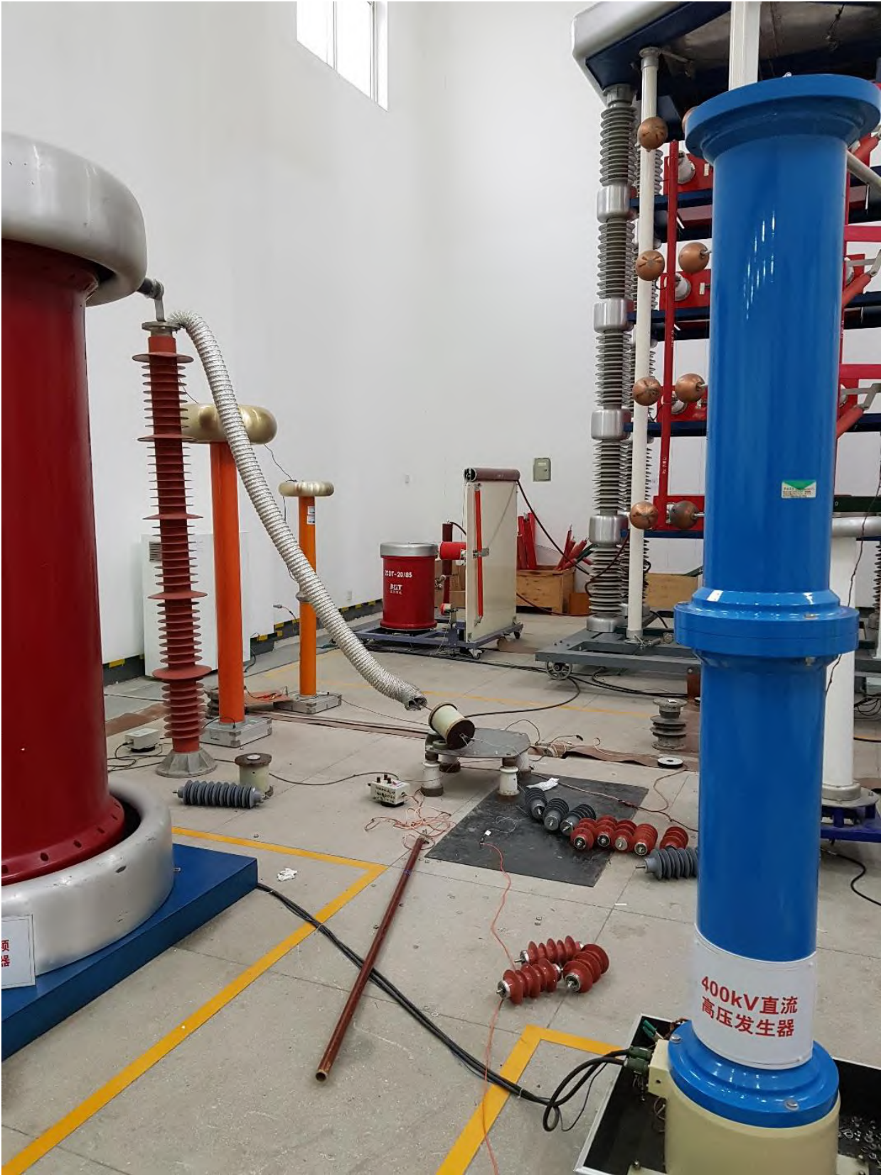
Object under power frequency voltage test
