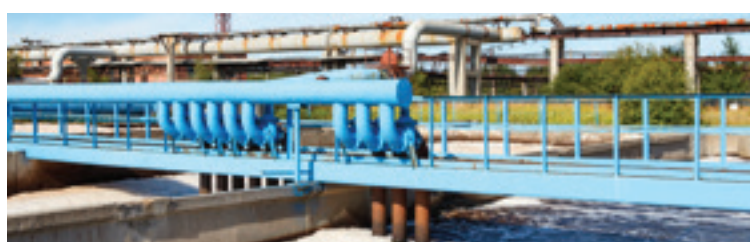
Waste Water Treatment Plant
