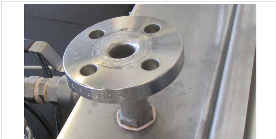
Figure 8 – Steam line connection
