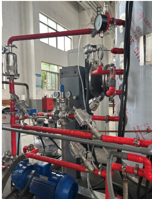
(Pipe insulation and chamber insulation)
