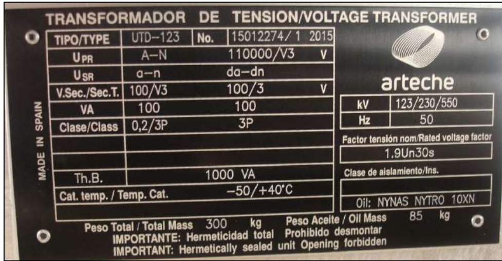
Picture 1.1 – Rating plate of voltage transformer.
