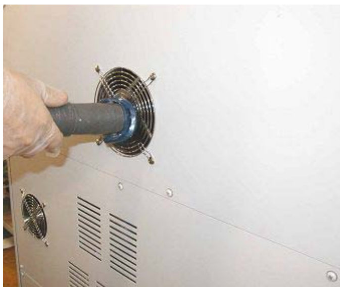
Cleaning the panel fan
