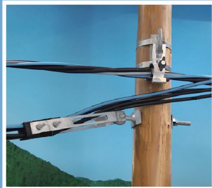
Self-supporting LV-ABC lines
