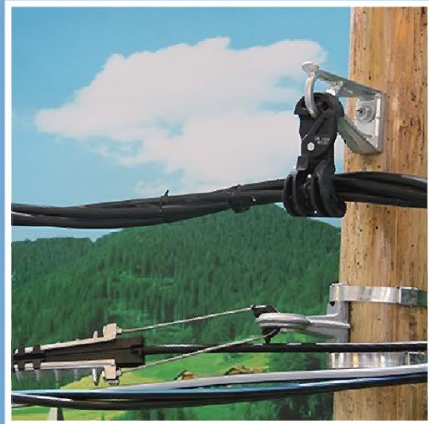
LV-ABC lines with insulated neutral messenger
