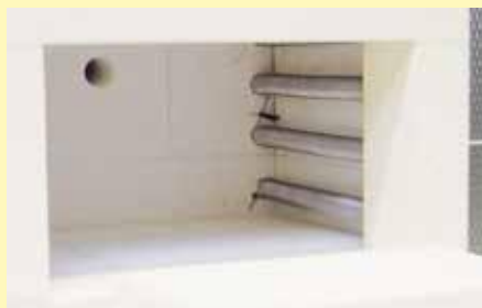
Furnace lining with high-quality lightweight refractory brick insulation
