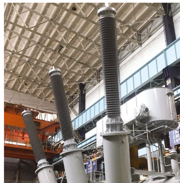
变压器套管安装在变压器上进行出厂试验 Installation of 550kV transformer bushing on the transformer for Routine test
