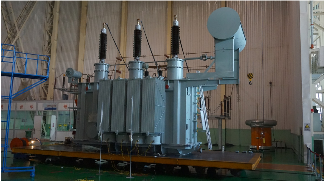
Transformer during the temperature rise test (ONAF)
