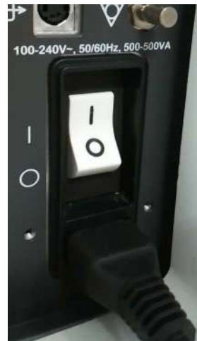
Figure 8-307 Turning on circuit breaker
