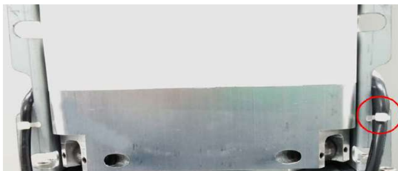
Figure 8-282 Cable tie point
