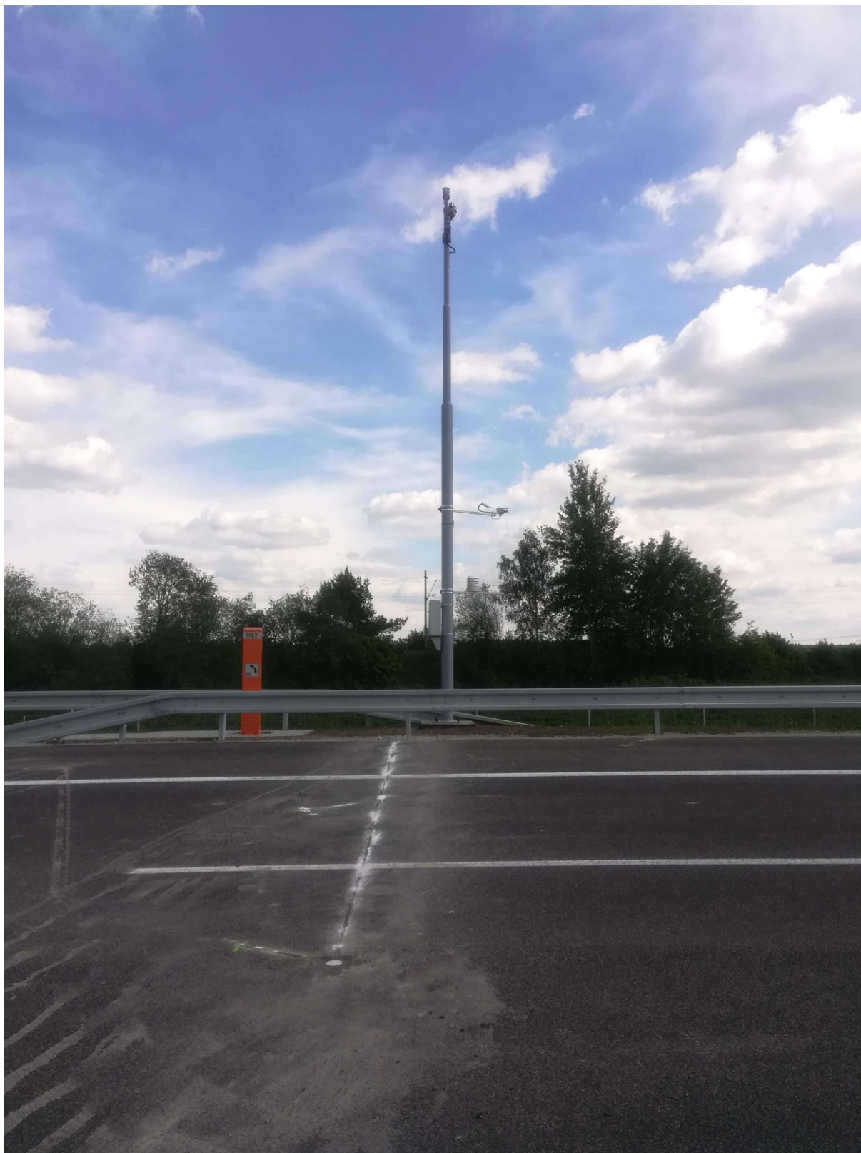
Fig. No. 15: Example of installation of road sensors for 2L with weather station and DIS SOS
