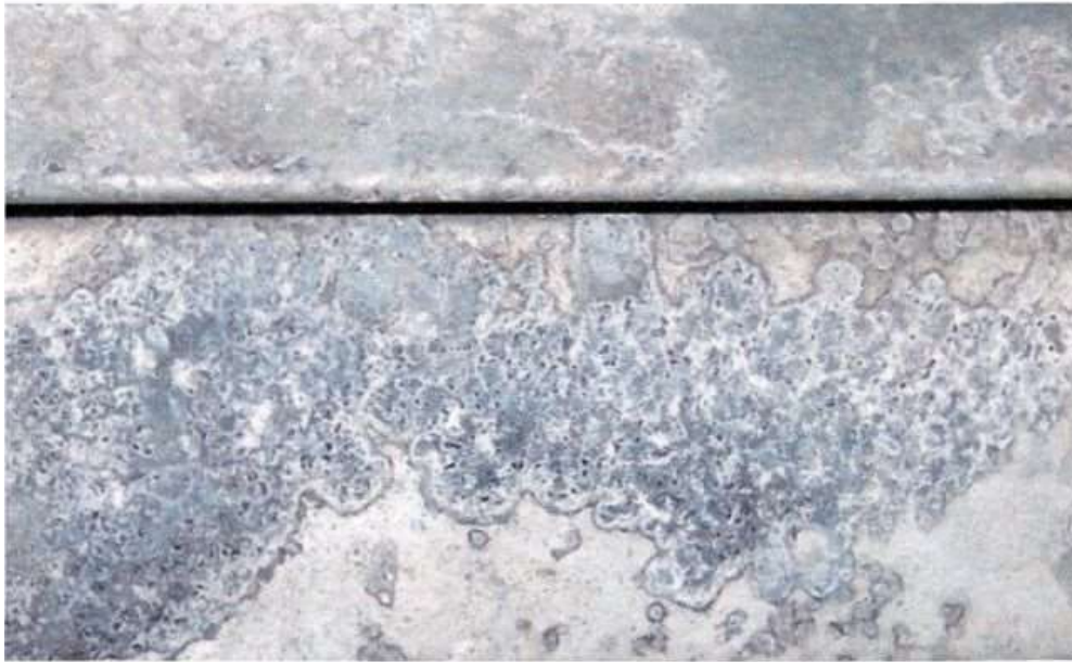
The surface of the hot-dip galvanised trailer, where white corrosion has developed, when the trailer has been exposed to road salt.
