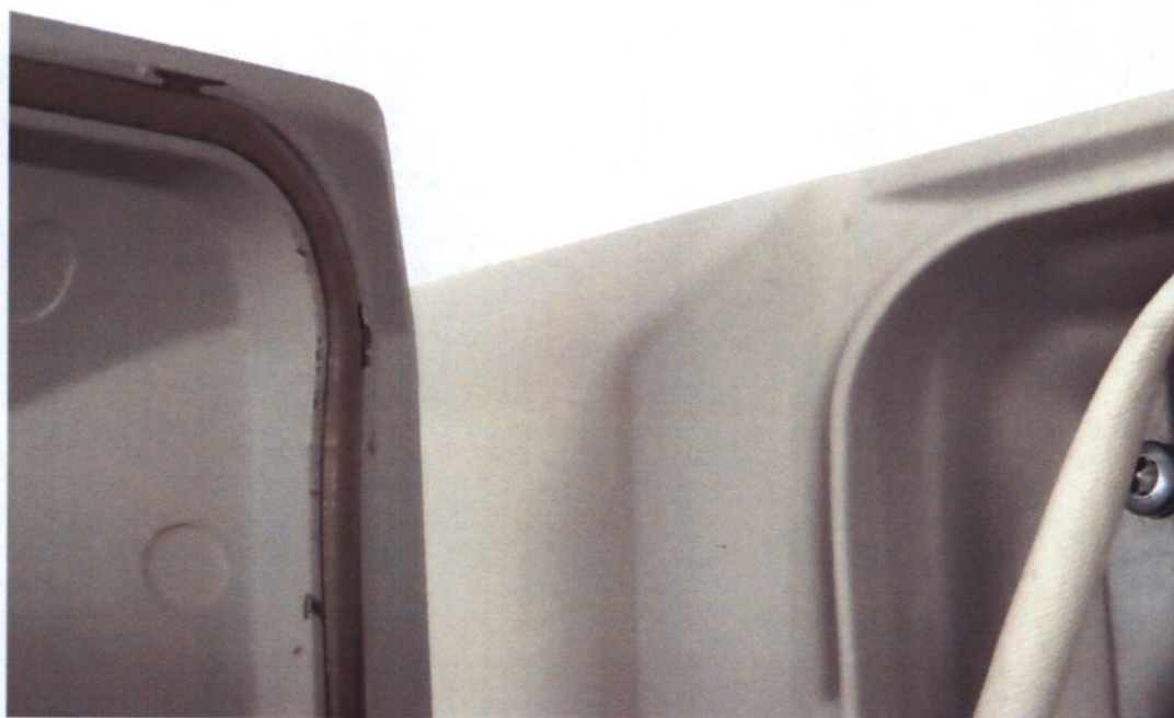
Fig. 5 - gasket of the luminaire
