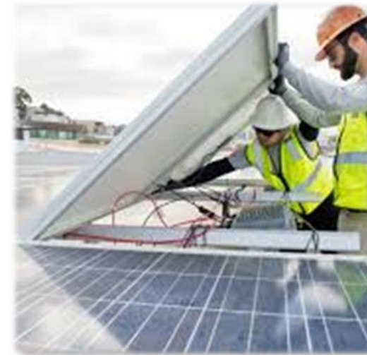
Maintenance Services for Solar Power Plants
