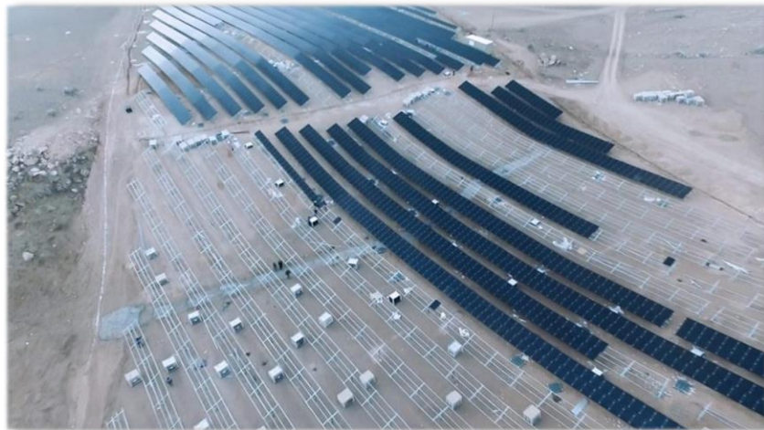
3650 kWp Solar Power Plant, Ankara / TURKIYE
