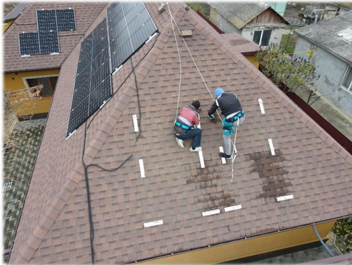
11.2 kWp Rooftop Solar Power Plant, Hinceşti / MOLDOVA
