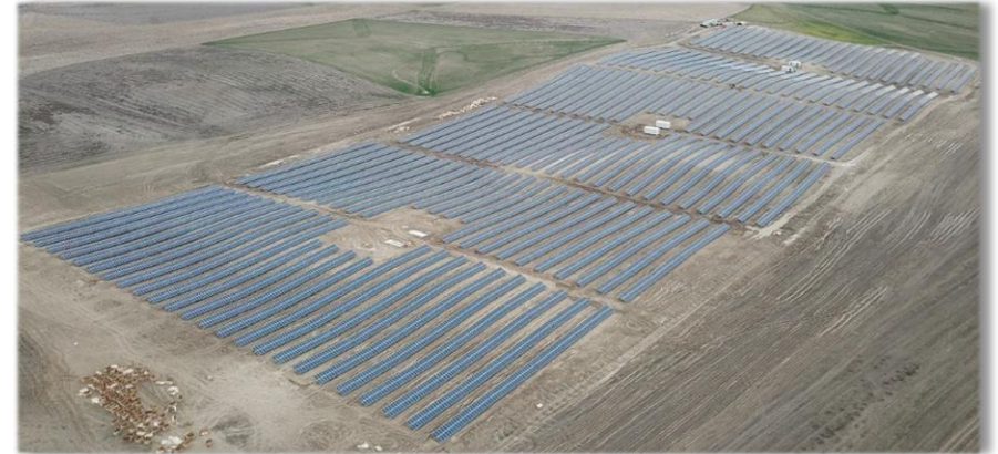
6980 kWp Solar Power Plant, Ankara / TURKIYE
