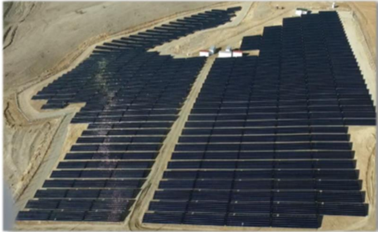
2245 kWp Solar Power Plant, Kırıkkale / TURKIYE
