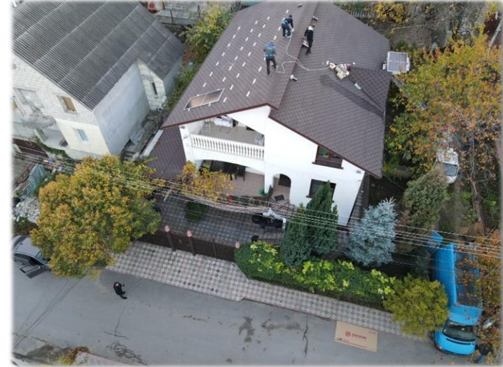
9 kWp Rooftop Solar Power Plant, Codru / MOLDOVA
