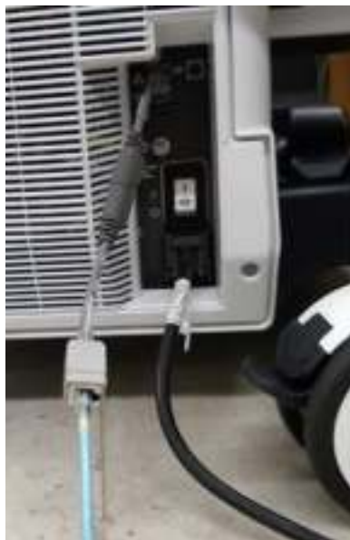
Figure 3-7 • LAN Cable with Protection Cable (Example)
