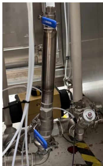
Figure 8. The collection system of leachates.
