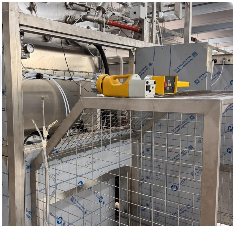
Figure 7. Device for aerosol sampling (SAS) positioned near the opening door of the sterilization chamber.
