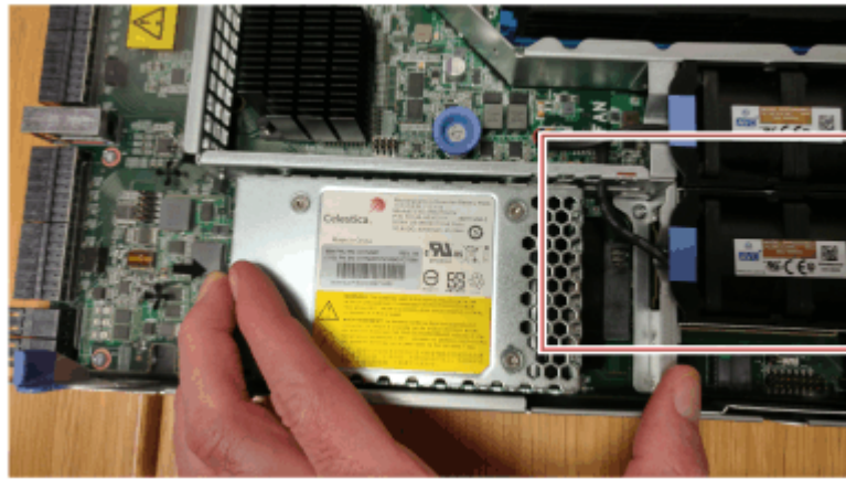
Figure 82. Replacing the node battery
