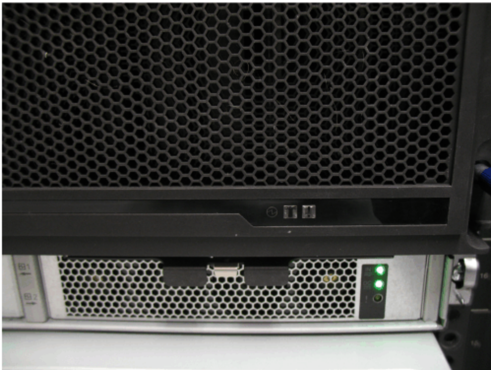
Figure 155. Power supply indicators
