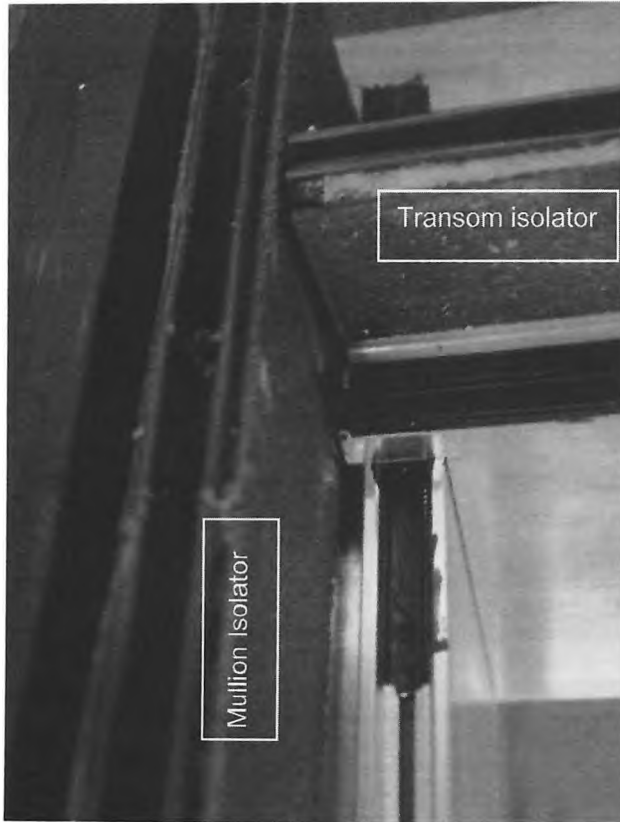
Photo 5 Rebate at removed pane, internal glazing gasket in mullion also removed
