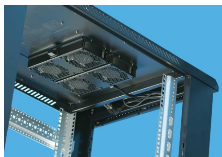
Inside view after installation
