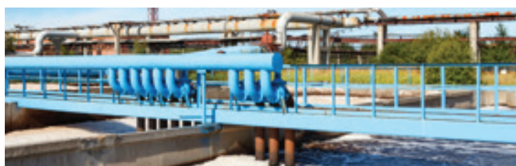
Waste Water Treatment Plant
