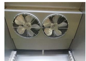
Detail of fans
