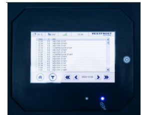
Remote alarm logs
