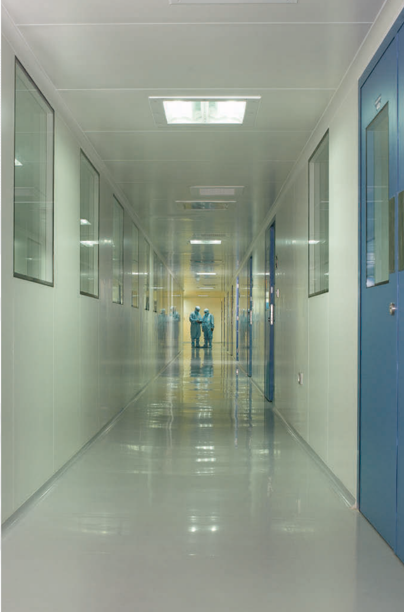
Ultra-modern Clean Room (Class 10,000) Infrastructure
