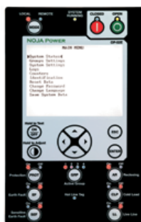
Autorecloser Control Panel
