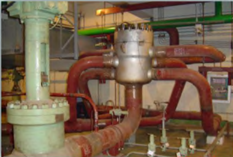
General view of the assembled CPHTD pump unit 850–400 A before installation of thermal insulation
