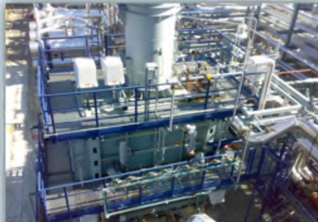
GPC system on IZOMALK-2 unit, JSC Gazpromneft – Omsk Refinery, 2011
