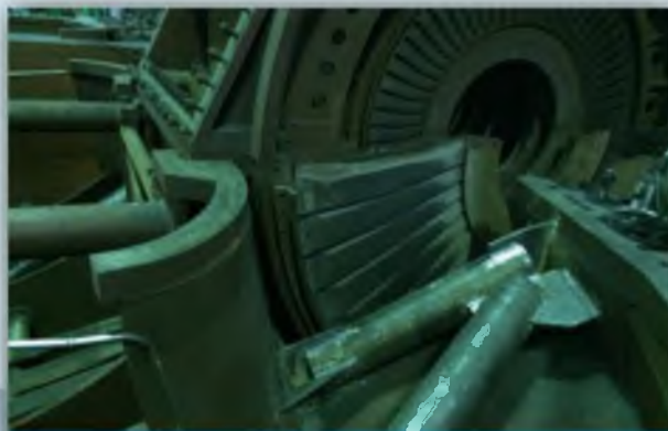
Reinforcing elements in exhaust pipes of the low pressure cylinder
