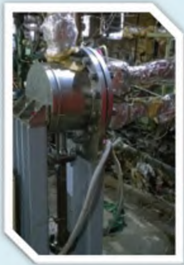
Gas blow-off processing system heat exchanger KKS 10KPL11AC002 with a stack of brazed plates Plate Stack XPSP 50 for the Belarus Nuclear Power Plant
