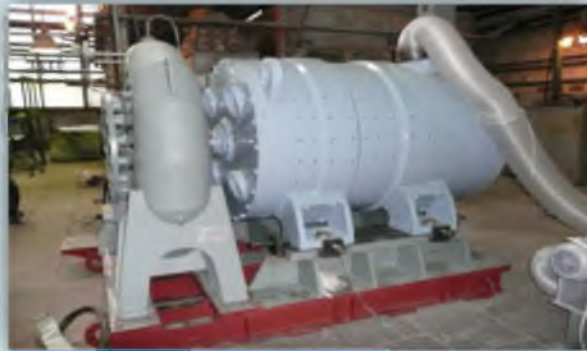
1.8 MW hydroelectric unit at Dzhradzor HPP (Armenia)
