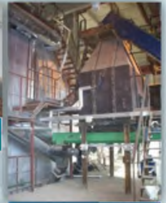
Feed bin with feeder
