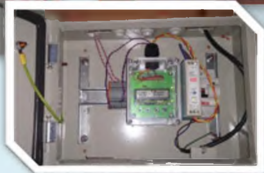
8. Test bed for checking operability of time-to-failure controllers
