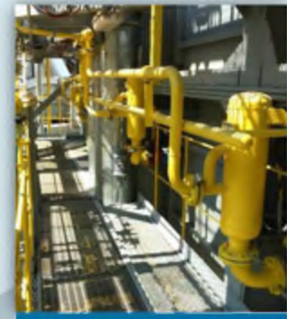
GPC system on the heat recovery boiler, LUKOIL Neftokhim Burgas AD, Bulgaria, 2014
