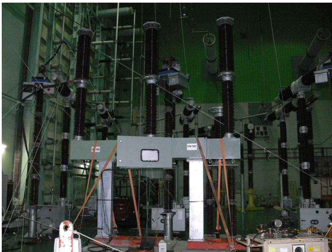
Photo. HP02 : After short-line fault tests
