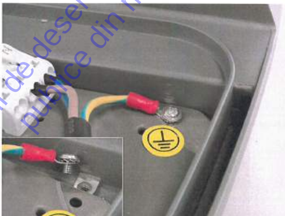
Protective earth on painted assembly plate
