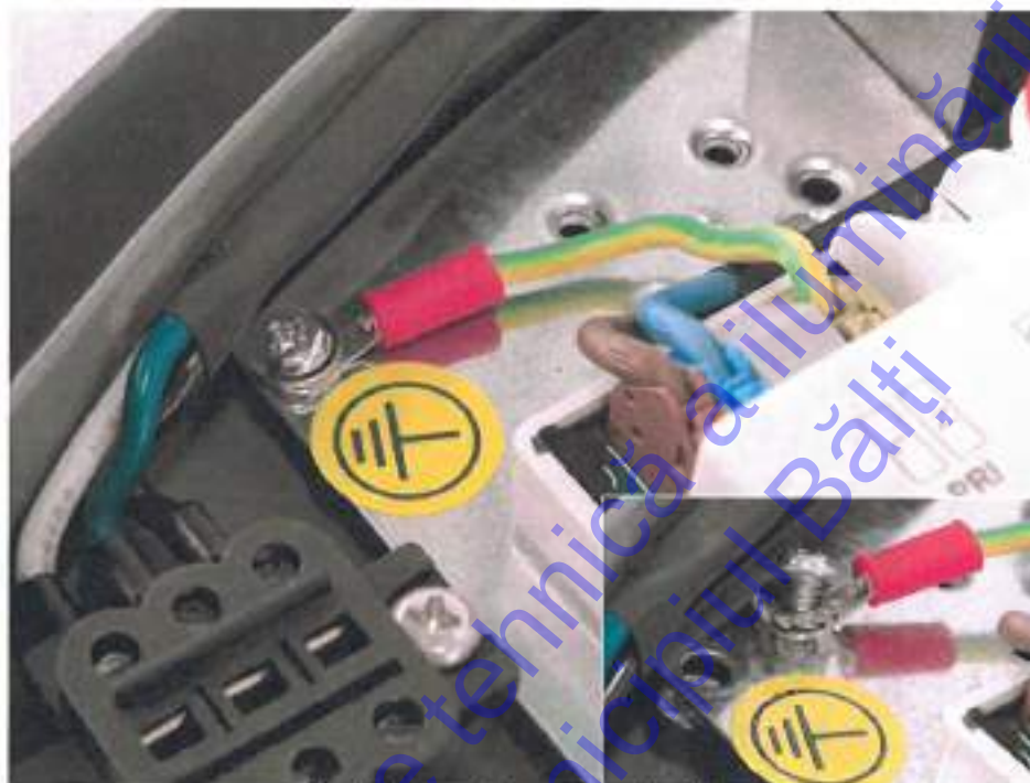
Protective earth on assembly plate
