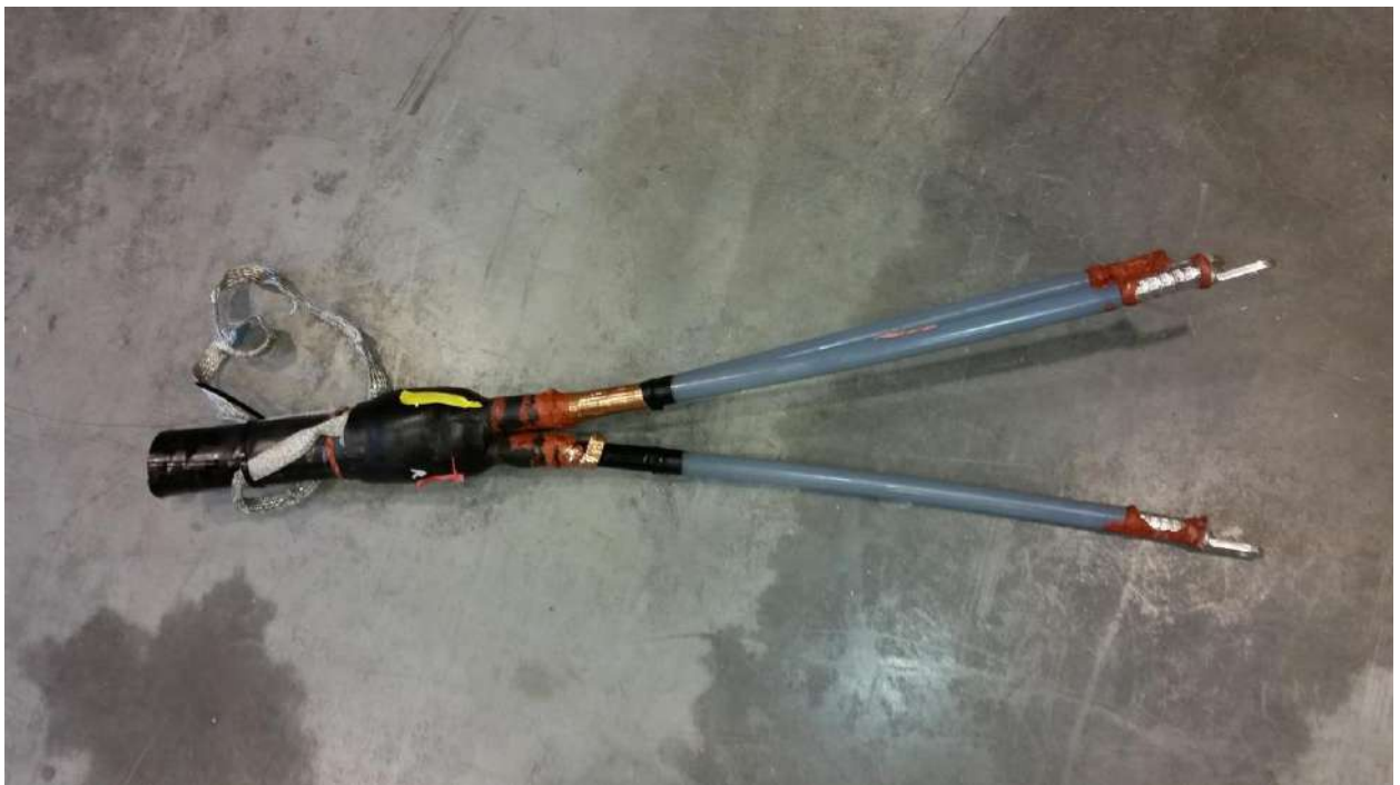
Indoor termination humidity sample
