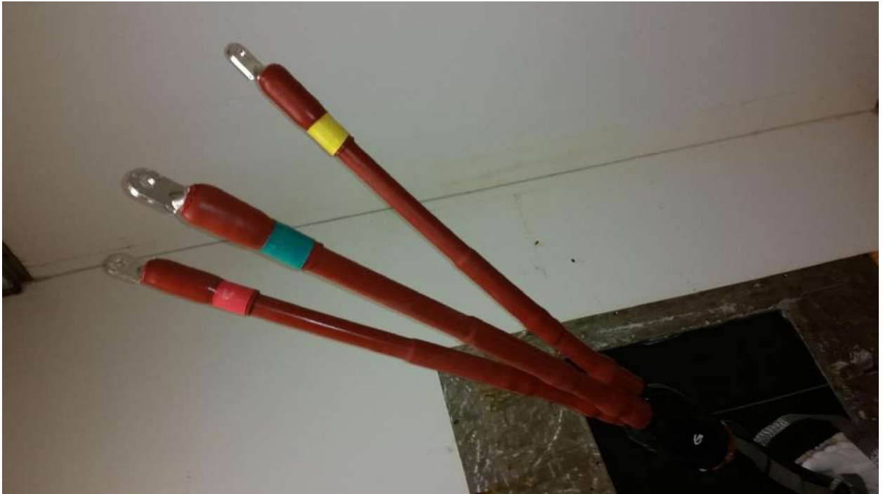
Indoor termination after test
