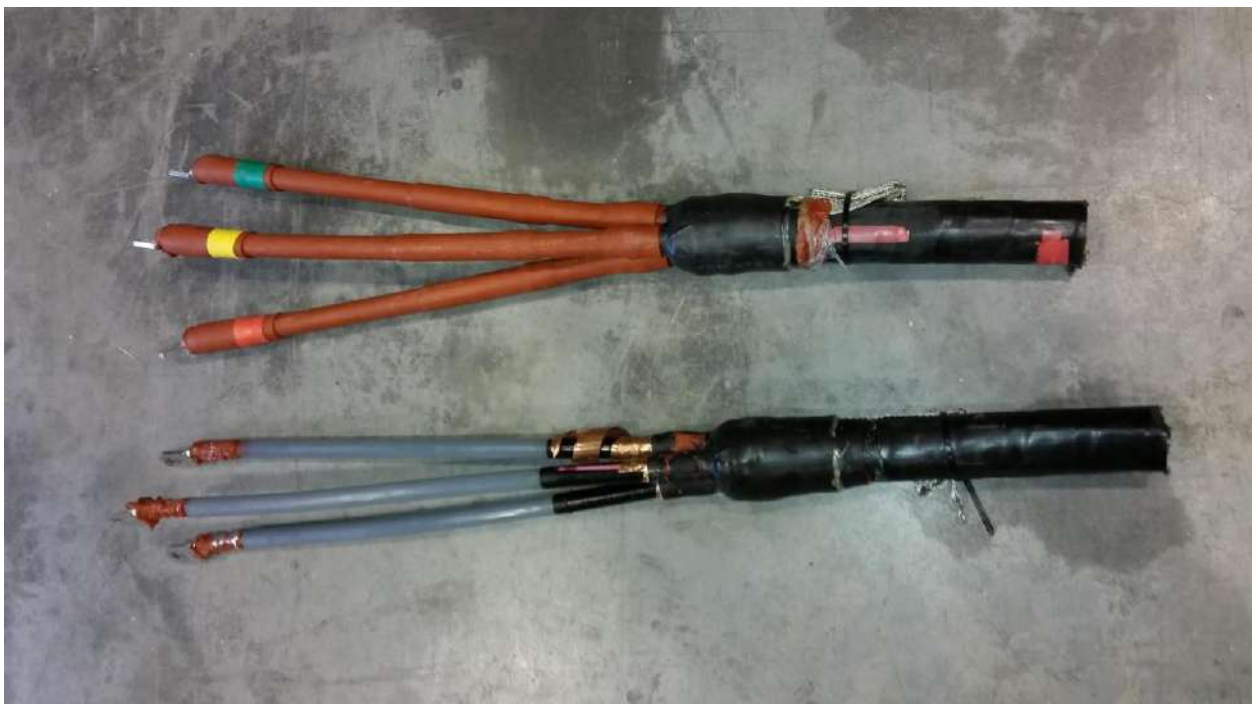
Two indoor terminations
